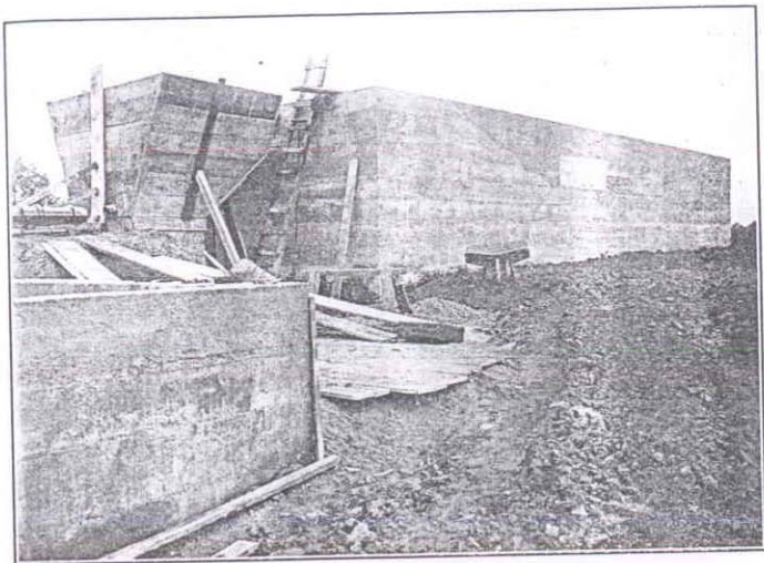
Burlington. Thomas Devlin Manufacturing Company. Septic Tank.
